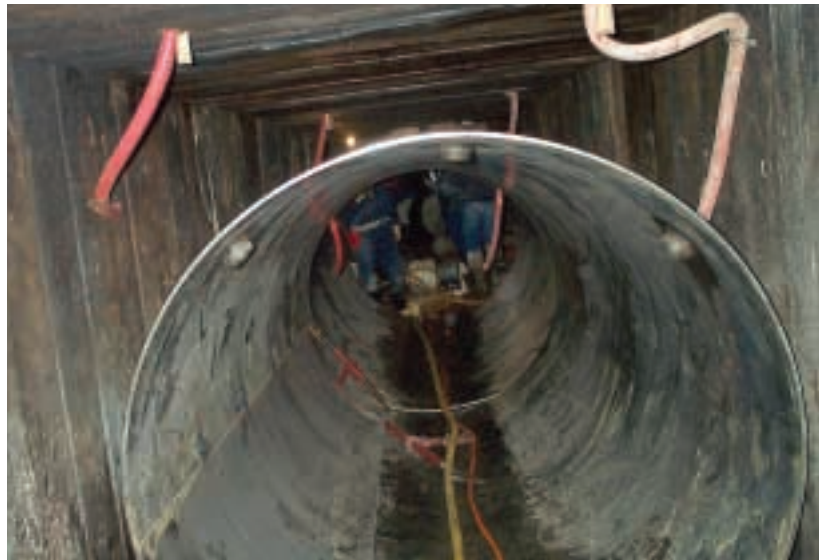
Above: Steel pipe being expanded inside the timbered section. Note the grout hoses reaching above the timbers
