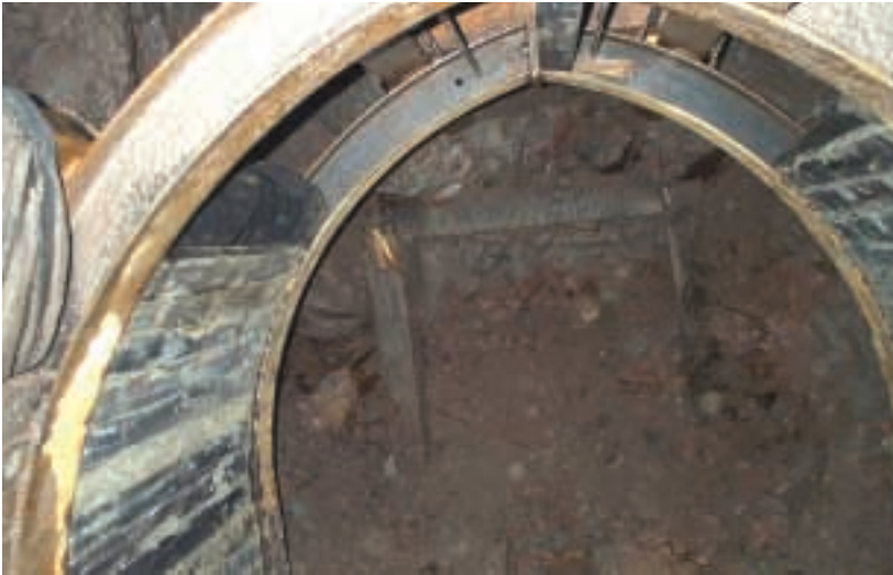
Above: View of the face while mining through the caved area. The timber set is clearly visible within the muck
